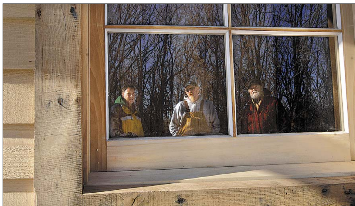
Peoria Park District employees Tom Miller, Tim Varvil and Dale Goodner look over the clapboard siding and new windows installed at the Sommer Park cabin.
