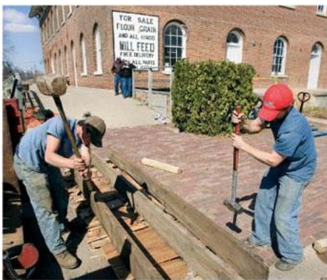
Ed Powell, left, and Ryan Owens of Trillium Dell Timberworks in Knoxville, Ill., beat sections of flooring apart during renovation efforts at the Wapsipinicon Mill in Independence. Floods damaged the historic structure. (RICK CHASE / Courier Staff Photographer)
